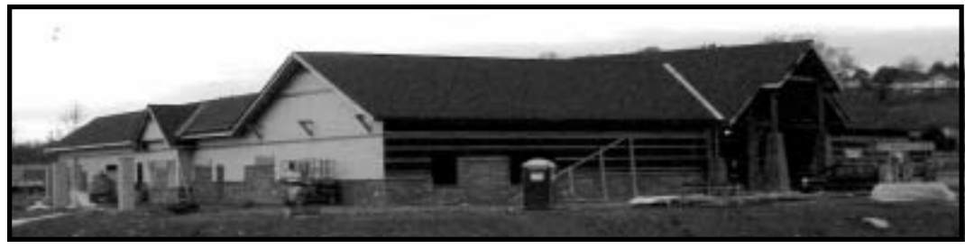
The Knoxville-Knox County Animal Center is 75% complete and on schedule to open in mid-January.
